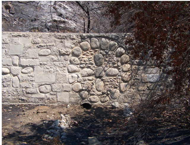
Figure 110: Stoppage Dam detail located off of Vista Del Valle Drive east of the Roosevelt Golf Course. View NE. Photo: ICF Jones & Stokes, June 2007.
