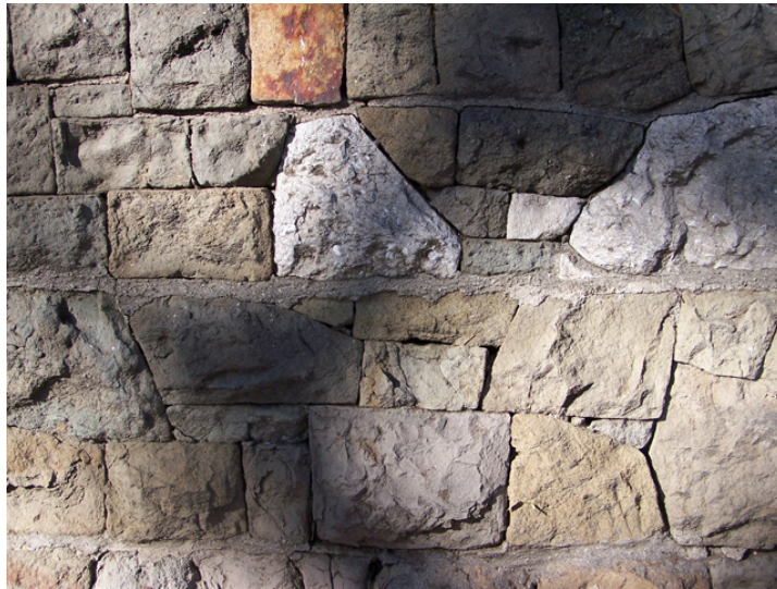
Figure 106: Barrier wall along Western Canyon Road due west of the Griffith Observatory. View N. Photo: ICF Jones & Stokes, August 2007.
