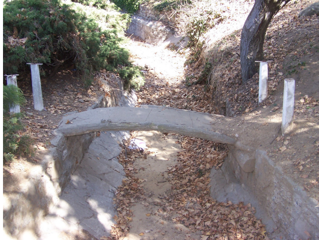
Figure 112: Drainage area with concrete bridge at junction of Camp Road and Griffith Park Drive, c.1935. View E. Photo: ICF Jones & Stokes, August 2007.
