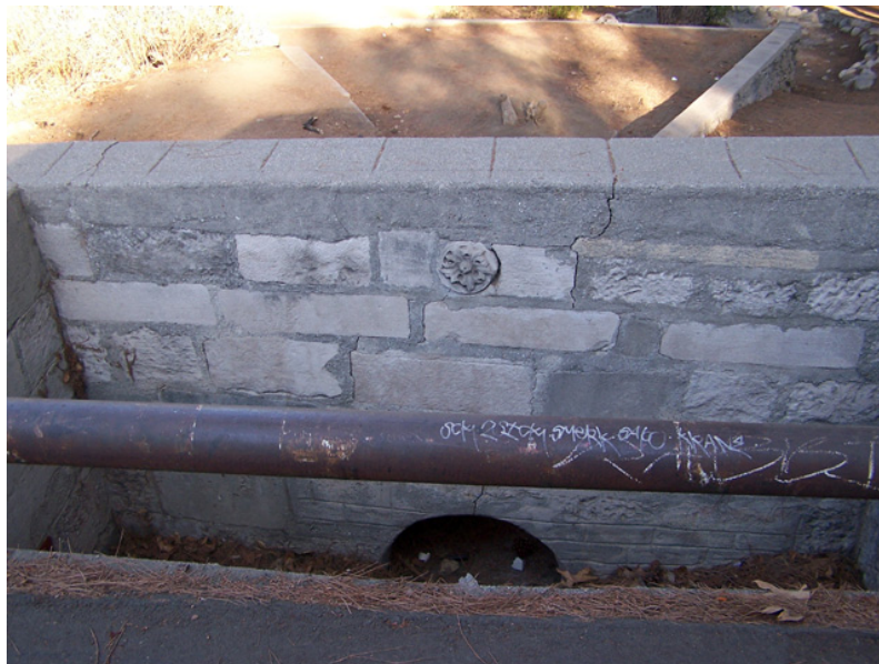
Figure 113: Drainage element with modillion, c.1935. View E. Photo: ICF Jones & Stokes, March 2008.
